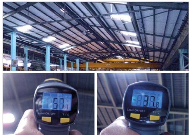
Hall roof inside (before-after): The temperature was reduced by 19.3°C. Use: Improved working conditions, energy saving, cost reduction of roof maintenance.
