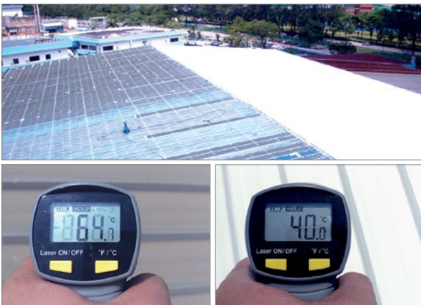
Industrial hall in Malaysia. Hall roof outside (before-after): The roof coating reduced the surface temperature by 24.7°C.
